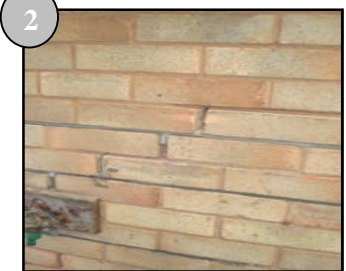
2 Helical bar crack stitch inserted and sealed in special grout ready for final re-pointing to hide repair.
