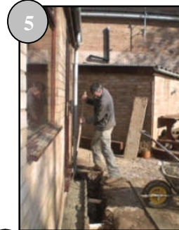
5 Concrete added to full length of the trench as specified on this particular job
