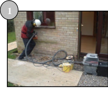
1 Cutting out of mortar joints for crack stitching using twin wheel diamond cutter and dust control vacuum.
