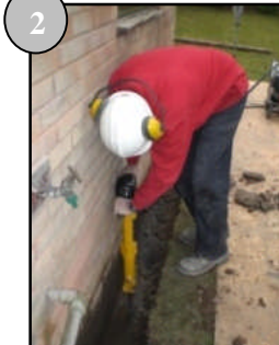
2 Concrete footings need breaking out for the concrete pile replacement.
